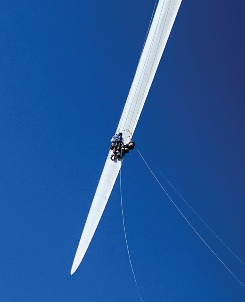
A technician repairs a blade at the Block Island Wind Farm. Photo: Andrew Ahern
